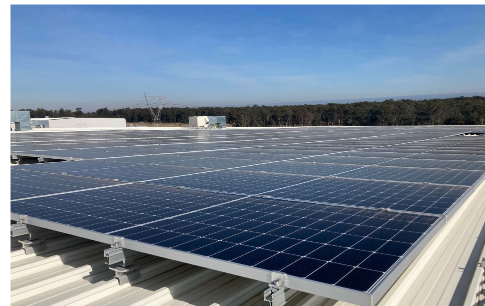
TJX Australia's processing center in New South Wales features rooftop solar panels and a Green Star certification.
